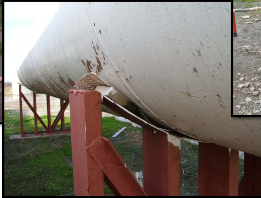
Improper Saddle Configuration
