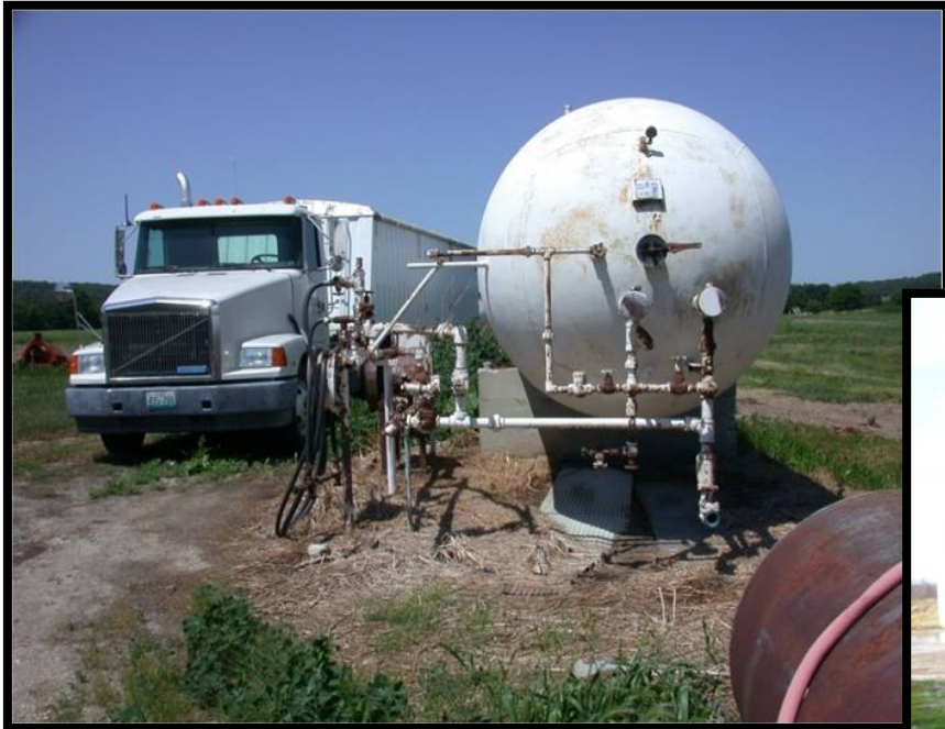
Insufficient/Nonexistent Vehicle Barriers
